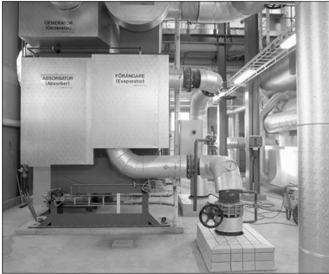
Figure 6.8 Using heat pumps. This large industrial heat pump is taking its heat from the flue gases from waste combustion at Vattenfall, Uppsala Energy. In the process the gas condenses and the heat extracted is transferred to the district heating system. In other large-scale applications heat is extracted from sewage water or surface water. The chilled water may be used for district cooling. Most heat pumps are smaller and used for individual homes. (Photo: Kjell-Arne Larsson)
