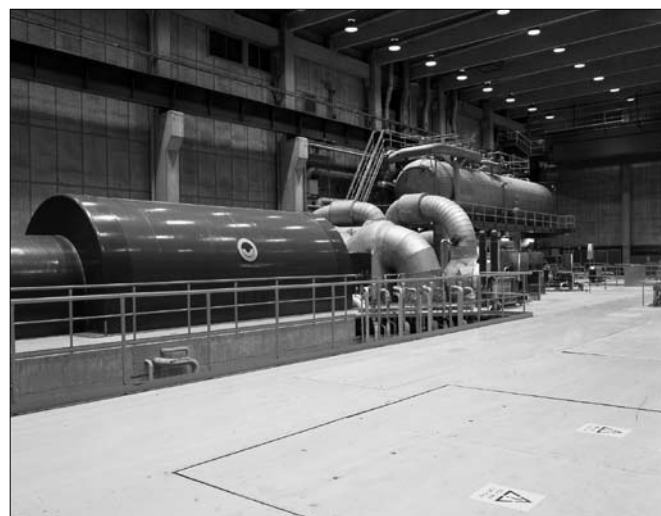
Figure 6.5 Cogeneration. Combustion for heat production may be coupled to electricity generation in turbines, as in this turbine hall. When the hot steam is pressed through the turbines electricity is generated. The steam is cooled to temperatures appropriate for the district heating system. With this combined system efficiency is close to the theoretical maximum. (Photo: Kjell-Arne Larsson)
