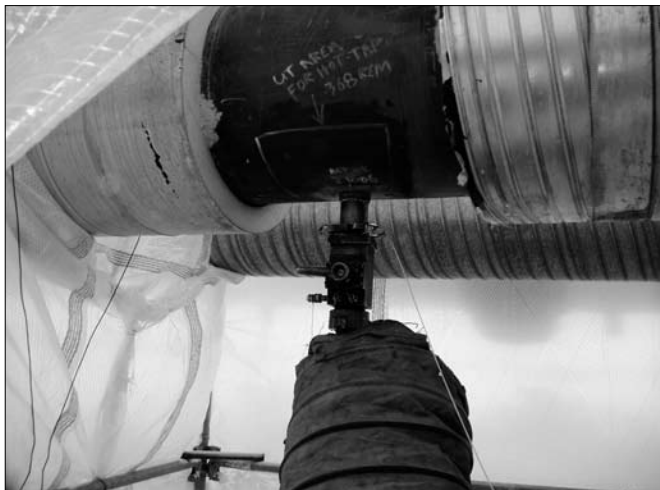
Figure 6.12 Energy efficiency requires that pipelines are well-insulated. See also Case Study 4. (Photo: Waska Williams Jr. – North Slope Borough)
