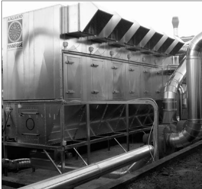
Figure 2.1 Sleeve filters air-cleaning system AAGAARD. Produced in Denmark, in 2001.
