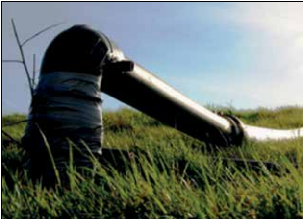
Figure 10.3 Extraction and transportation of landfill gas from the landfill body.
