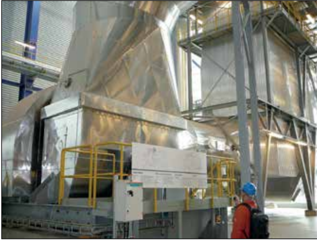
Figure 16.3 Powerful and effective electrostatic filters have been installed at the incineration plant SYSAV, Malmo to clean and catch harmful emitted gases.
