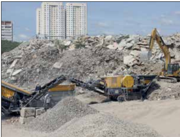
Figure 17.1 Processing of construction waste (reinforced concrete) at the crushing plant. The processed material (rubble) will be used for road construction.
