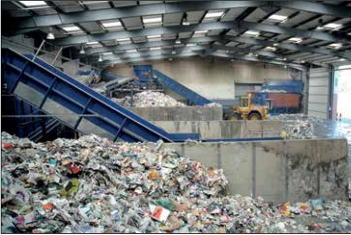
Figure 5.5. Automatic waste sorting station in Hamburg, Germany
