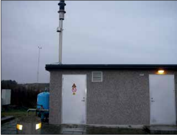
Figure 16.7 The landfill MERAB near the Swedish town of Ronneholm produces energy for its own needs from the collected landfill gas; this energy is also used for the common network. The roof of a small-scale generator installation is equipped with the burner for the post-combustion of flue gases.
