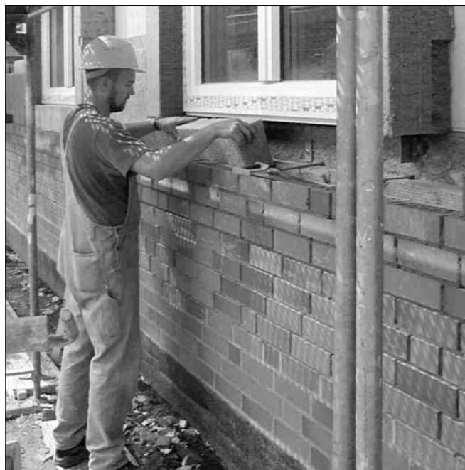
Figure 3.3 Building of a passive energy house. The house is insulated to achieve a U-value that does not exceed 0.15 W/m 2 K (0.026 Btu/h/ft 2 /°F) which typically corresponds to 20-40 cm of insulation.
